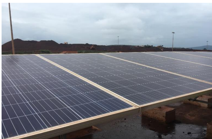
Figure 6: Solar PV Modules Installed at Mine
